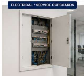
ELECTRICAL / SERVICE CUPBOARDS Show any electrical cupboards, DB boards, or service rooms nearby.
